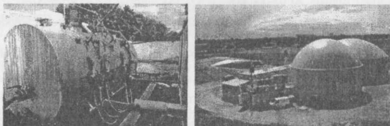
36-rasm. Biogaz qurilmalari
